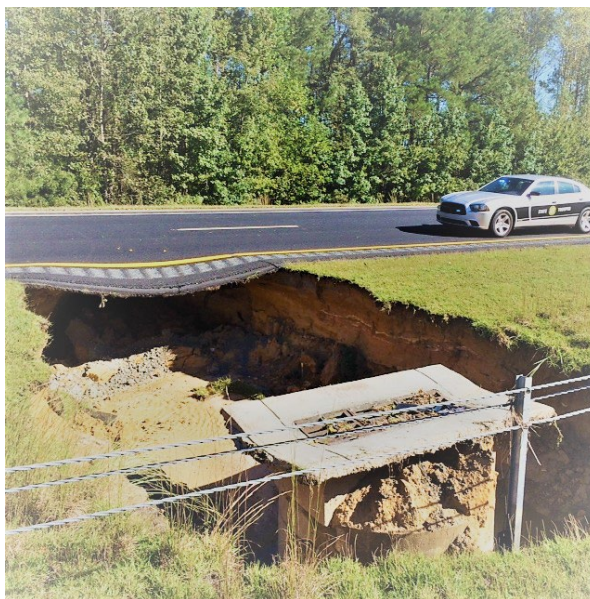
FIGURE 5.16: SINKHOLE IN NORTH CAROLINA
